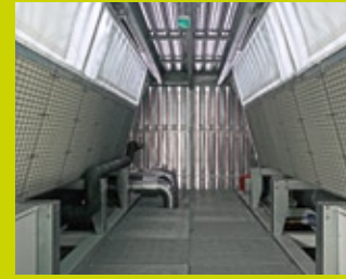
Air cooled chillers.
